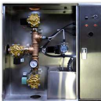
PCU CORE Control Panel
